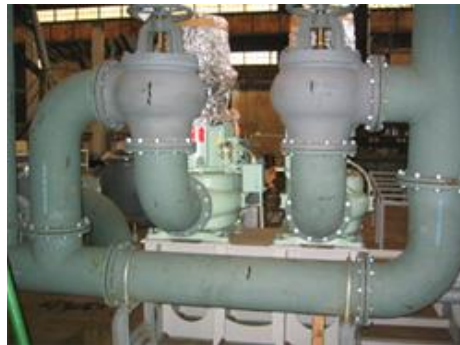
Piping in a ship
