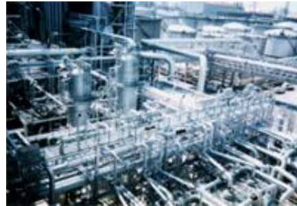
Stainless steel piping in a
